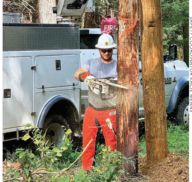
CHAINSAW SAFETY: United Electric Apprentice Lineman Spencer Pomerleau cuts an old pole with a chainsaw after setting a new one. Personal protective equipment is a must while operating a chainsaw.
