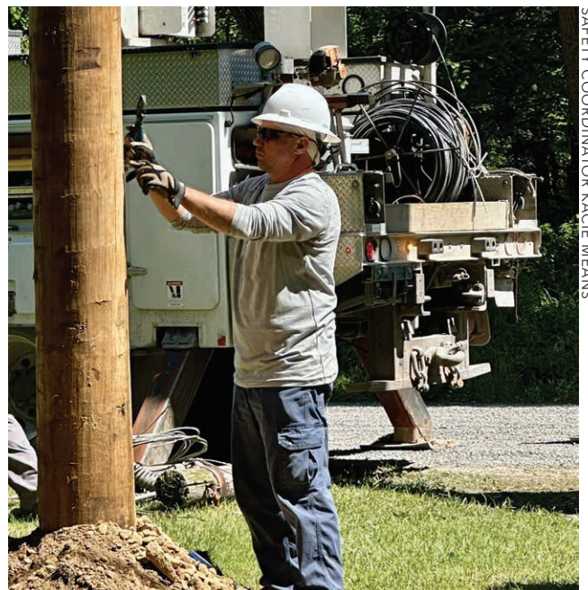
FINISHING TOUCHES: Crew Chief Chad Guaglianone installs United Electric's identifying pole tag after a new pole is set.
