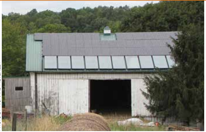
HOME OF CREAMERY: This 1880s-era barn is now the home of Cherish Creamery's dairy. Solar panels interconnected with United Electric's system are installed on the roof to provide some of the power needed to operate the creamery.
